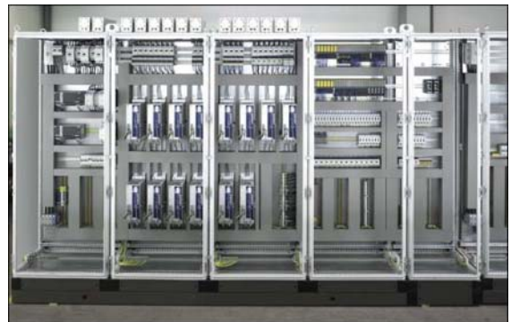
Picture 3: Switch cabinet with WATT inverters P6000
