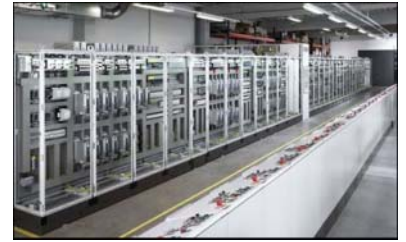
Picture 1: Switch cabinets
