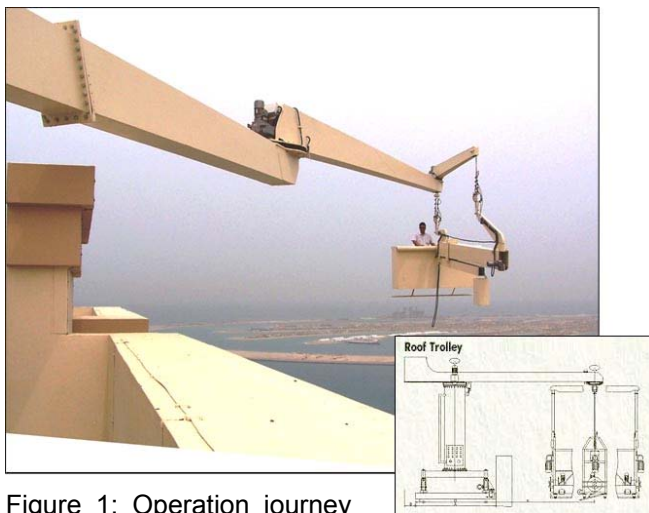
Figure 1: Operation journey of a facade lift in Dubai
